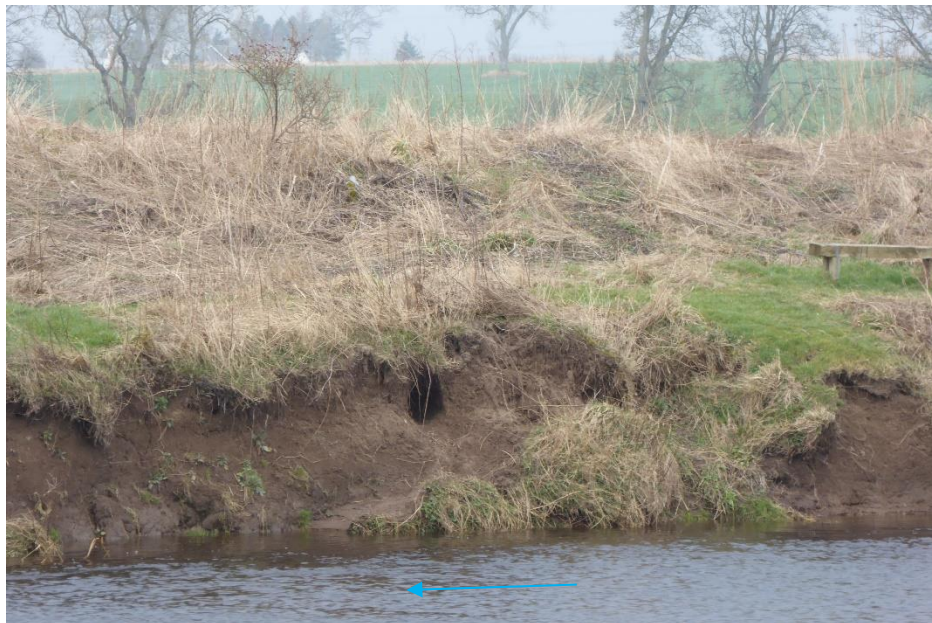
Figure 8. Animal burrowing on eroding bank. This can contribute to localised bank erosion during flood events when water flows into the open burrow saturating and collapsing the roof, causing the bank surface to slump.
