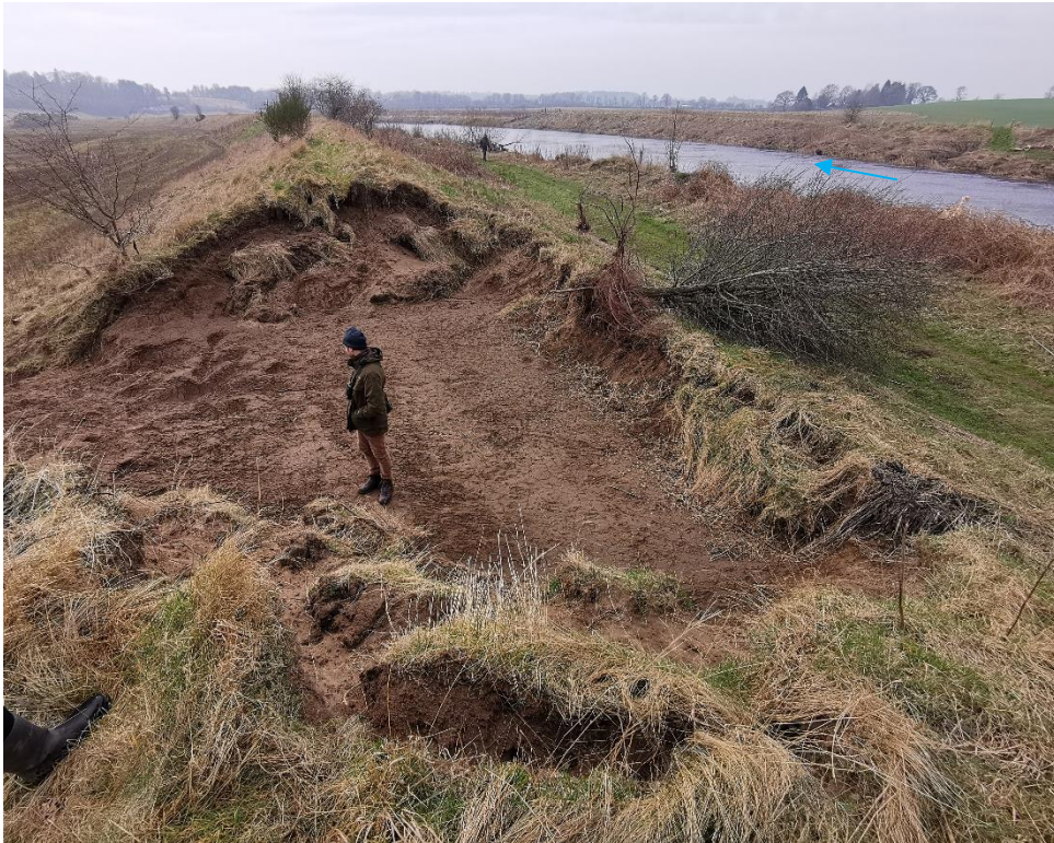
Figure 7. Example of embankment ‘blow out’ on the River Isla, this could have been caused by a combination of factors – embankment crest-overtopping by flood flows leading to scour on the landward side of the embankment and the weak bank materials used to construct the embankment. Beaver burrowing is less likely to have contributed to this embankment blow out due to the position of the embankment being set back from the river channel (>20m) and the shape of the scour hole on the embankment on the landward side.
