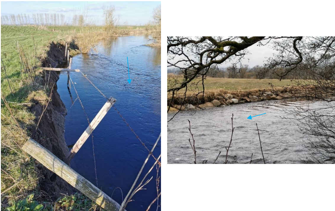
Figure 10. Left - river bank erosion on outside of a meander bend, fence line is on the top of the bank and has been undermined. Right – example of bank toe reinforcement using large boulders ‘rip-rap’, this does not stop erosion but leads to excess bank erosion downstream where banks are not protected.
